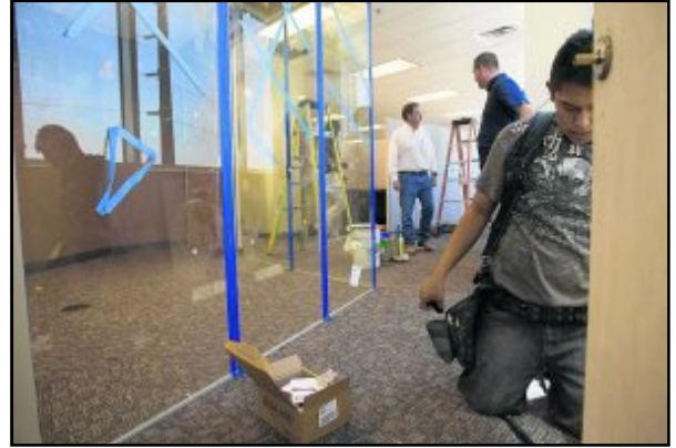
Contractor Lamorre Hobbs, front, installs door hardware while Unicon CEO John Blakley, left, and Jason Lacy, vice president of sales, look over the company's new office in Gilbert's Rome Towers. Unicon has leased 10,000 square feet on the fourth floor
