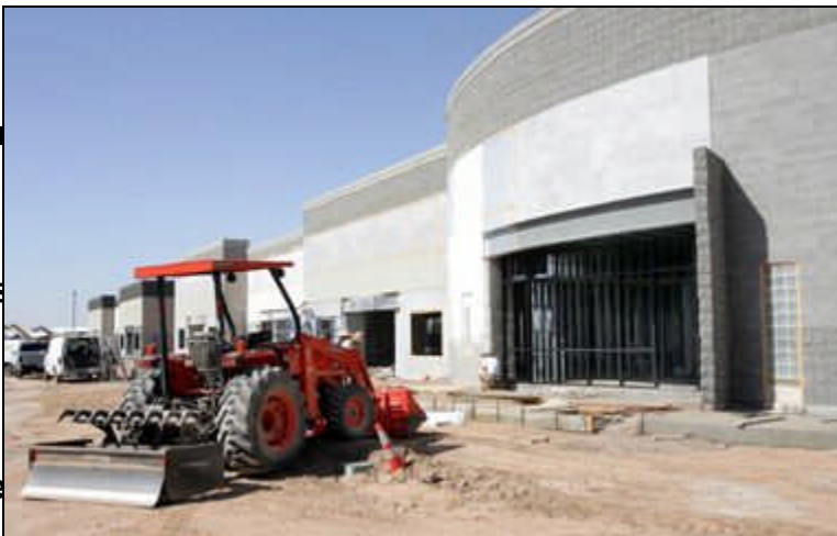
Staff photo by Steven King, Construction of some industrial condos is proceeding near Casa Grande Municipal Airport.
